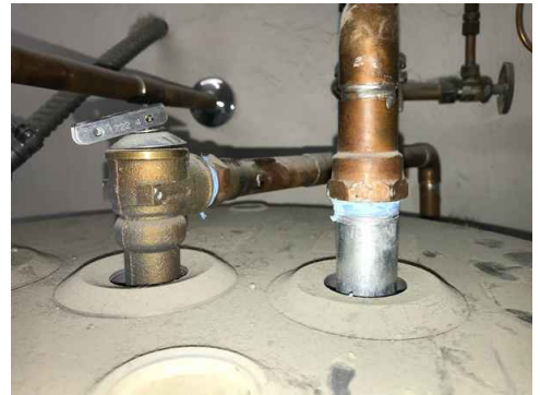
TPR Valve With Drain Line
