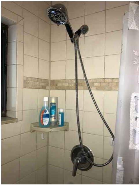
Spare Bathroom Shower
