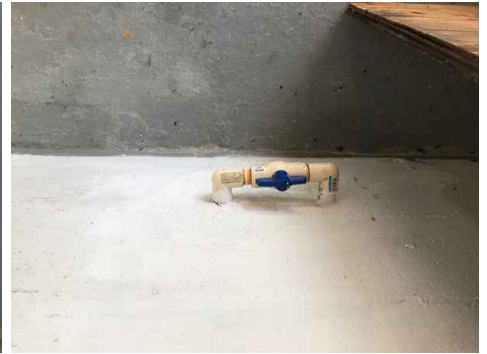
Shutoff valve garage
