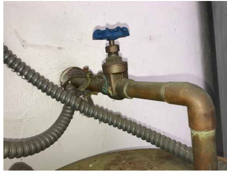
Hot water tank shutoff
