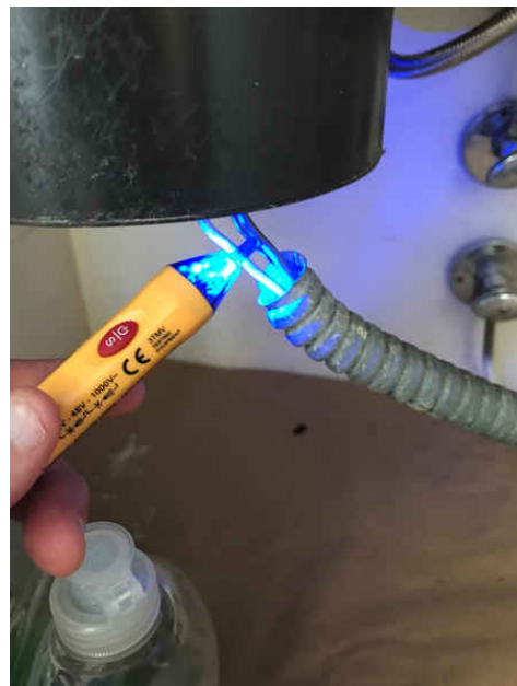
Wiring shows disconnected power
