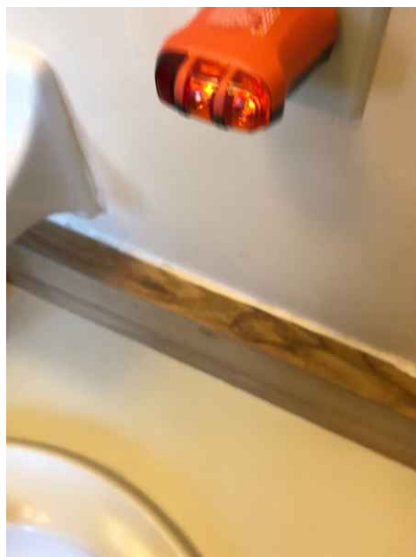
Outlet grounded properly
