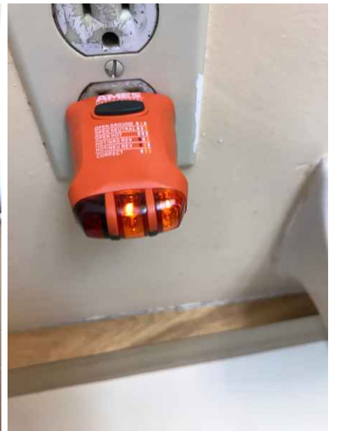
Outlet grounded properly
